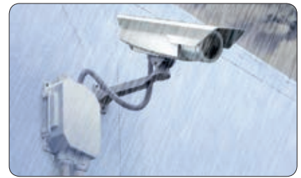
Installation with free cables.
